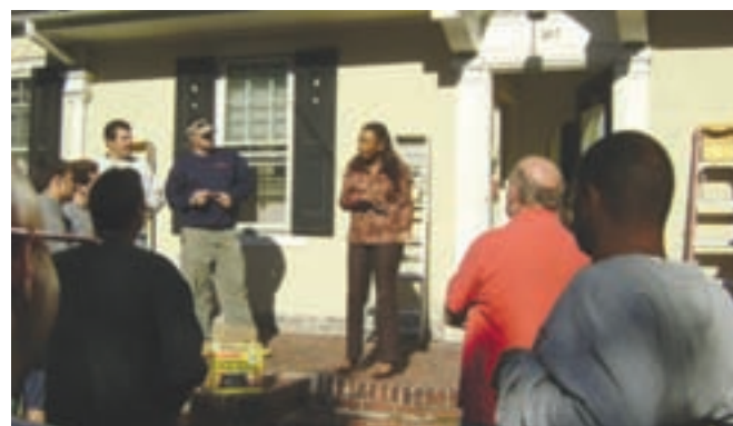
School House Lane Group Home for Girls was the site of the 16th Annual United Way Days of Caring. FAMECO Real Estate employees teamed up with A & E Construction to provide an extreme makeover for the Home's interior and exterior. BCS YES! Board member Carole Davis was on hand to welcome the United Way and workplace volunteers.
